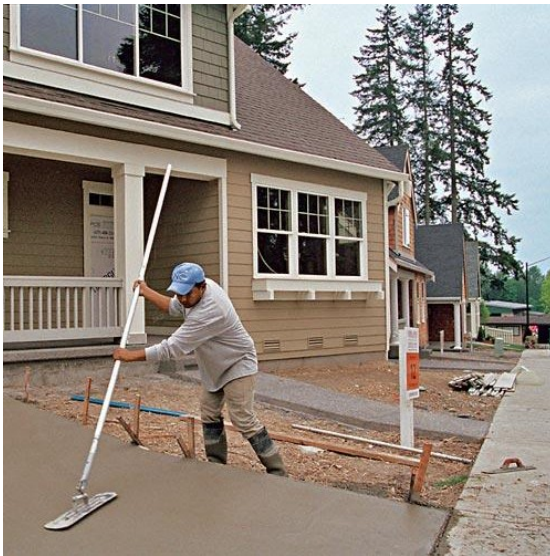
A driveway to a single-car garage is finished at Kirkland Bungalows, where 15 homes of approximately 1,500 square feet each are clustered on 2.2 acres and sell for about $450,000 each.
